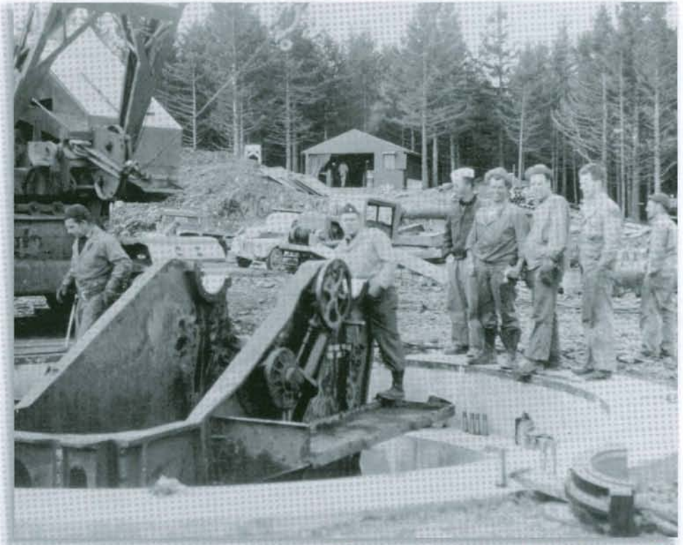
Seabees preparing to install 8-inch gun at Fort Abercrombie. 1943. (Kodiak Historical Society)
