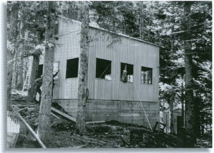
Radar station under construction at Piedmont Point, Fort Abercrombie. August 1943. (Kodiak Military History)
