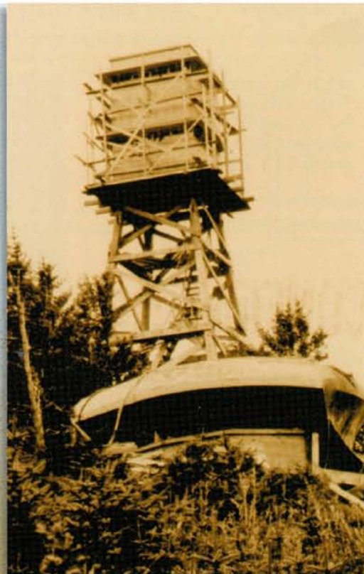
Under construction, this observation post at Miller Point, Fort Abercrombie, was a two-level wooden tower standing 50 feet tall. The gun battery command station was on the lower floor; base-end stations were on the upper floor. October 1941. (Kodiak Historical Society)
