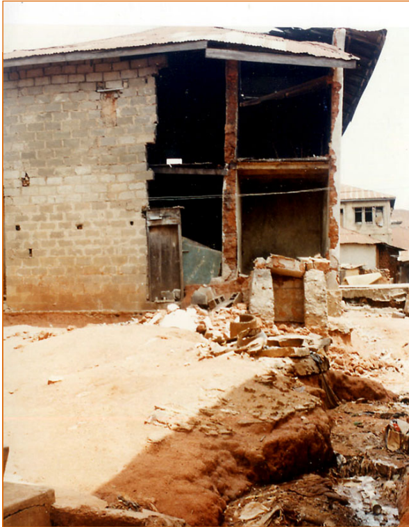
Photo 8 : Derelict houses in Bere, lack of drainage and appropriate waste disposal
