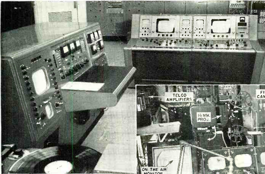
← Close-up of transmitter control console (left) and video console (right, center). The turntable in foreground belongs to sound desk. The video mixing desk operator faces the TV and audio racks which line wall behind the console in right center. Instruments enable operators to set and maintain proper audio and video levels of the signals feeding into the transmitter unit.
